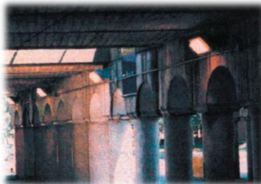
Obscured Sign at Metra Station Exit
